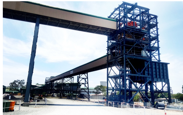
STRUCTURAL, MECHANICAL, PIPING, & PLATEWORK (SMPP)
