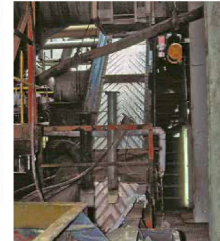
Chain conveyors are effectively protected with ABRESIST, KALOCER, KALMETALL or KALCRET
